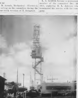
NEARING COMPLETION at the time this picture was taken is Lago's radio antenna, part of a new radio set-up that will connect Lago's Marine Department directly with Creole's Ammay Bay Marine Department. It will be used mostly to contact the Marine Department and the coordinator of cruise shipments in Venezuela. At present, Lago is waiting for its transmitter equipment. In the meantime Lago has borrowed a set from Creole.
